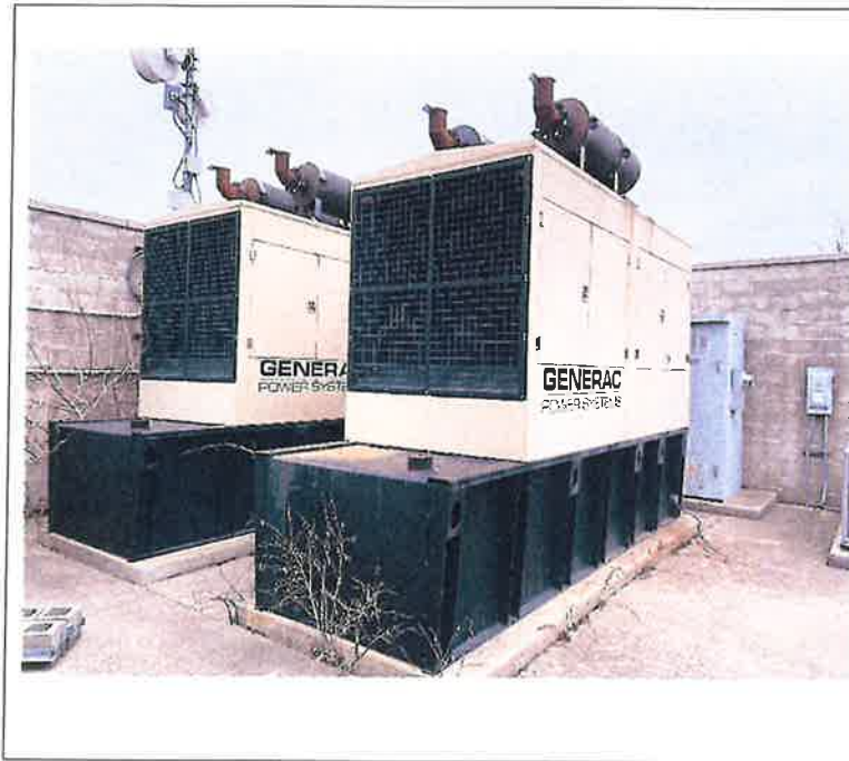
Two (2) 2005 Generac Model 5355210100 500kW Diesel Generators
